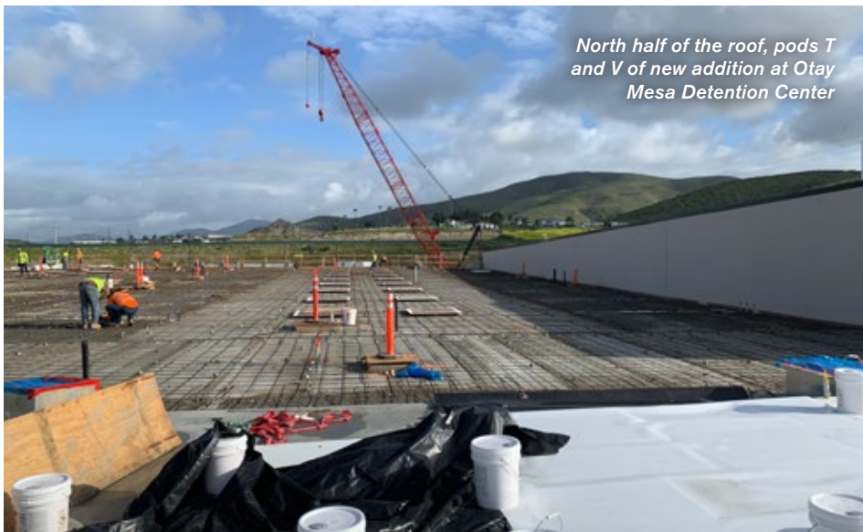
Northwest corner of the 512-bed expansion at Otoy Mesa Detention Center. The precast concrete building structure is now complete and work continues on the roofing, concrete floor slabs and the rough-in of interior mechanical and electrical systems.
