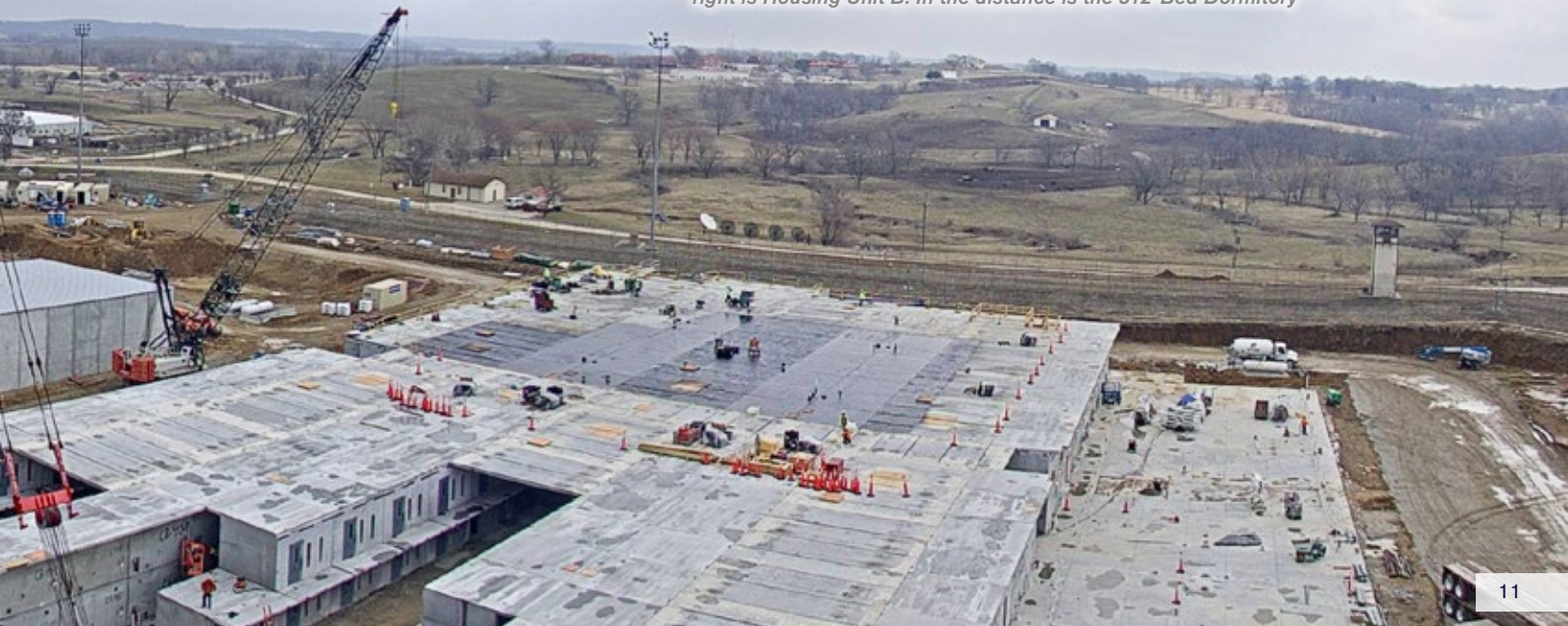
Four new buildings of the Lansing Correctional Facility construction. On the left is Housing Unit A (concrete slab underway), the center is the Support Building (medical, food services, recreation, spiritual life and staff support), and on the right is Housing Unit B. In the distance is the 512-Bed Dormitory
